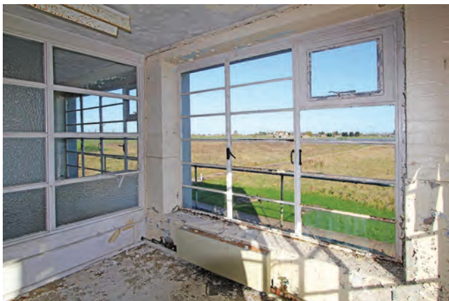
View across the airfield from the control room. 'P' site can just be made out in the distance
